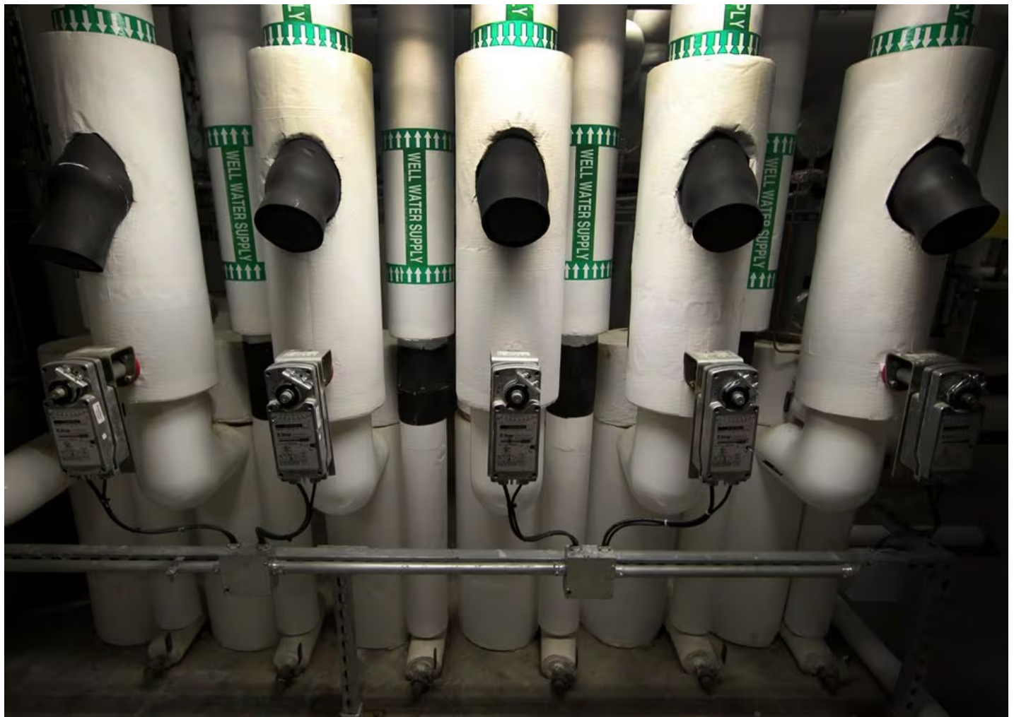
The pump room at the Isabella Stewart Gardner Museum, where geothermal well water is pumped, filtered, and reclaimed. DAVID L. RYAN/GLOBE STAFF
